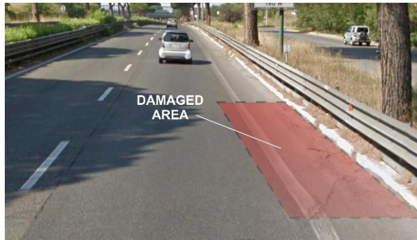
Fig. 1 – An example of asphalt damage due to the uplift of tree roots at the edge of the lateral lane and at the verge
