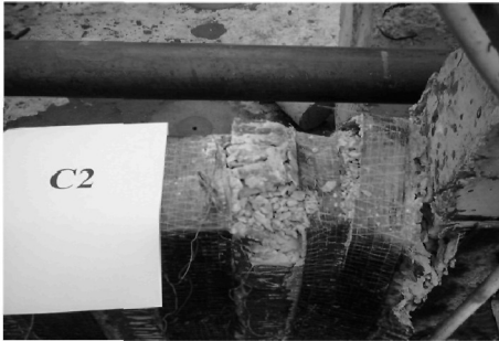
Figure 10 Failure of Specimen C2
