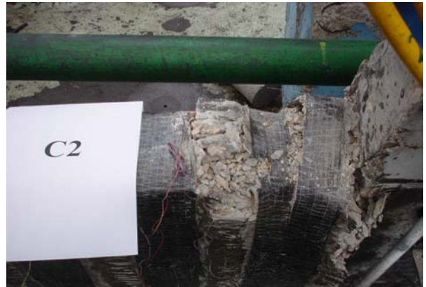
Figure 6 Failure of column C2
