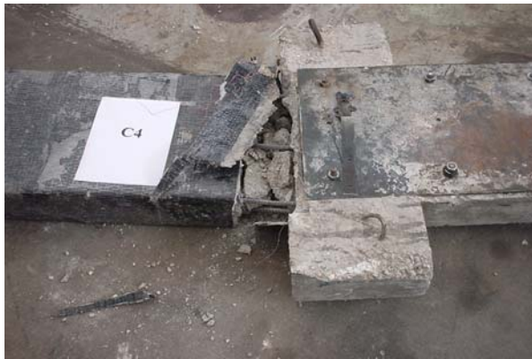
Figure 7 Failure of column C4
