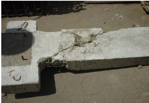
Figure 5 Failure of column C1
