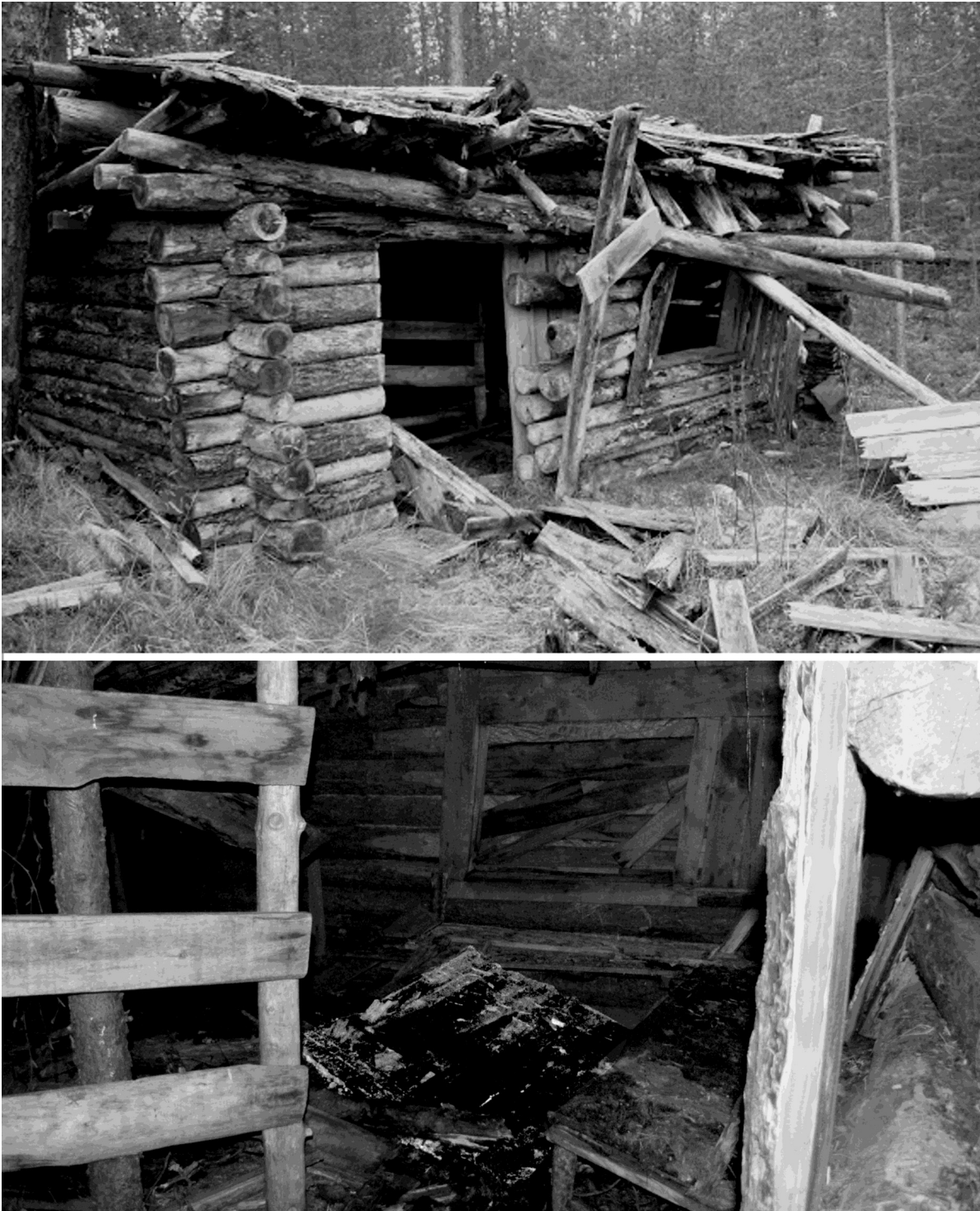
Figure 5. “Nangujärvi Saiholompolo”: top, a well preserved guard house before its roof collapsed in the winter 2011 (Photograph: Jari Leskinen / the Lapland Society for Military History); bottom, interior view of the guard house, showing the remains of bunk beds on the left, collapsed table in the middle, and benches along the walls (Photograph: Oula Seitsonen).
