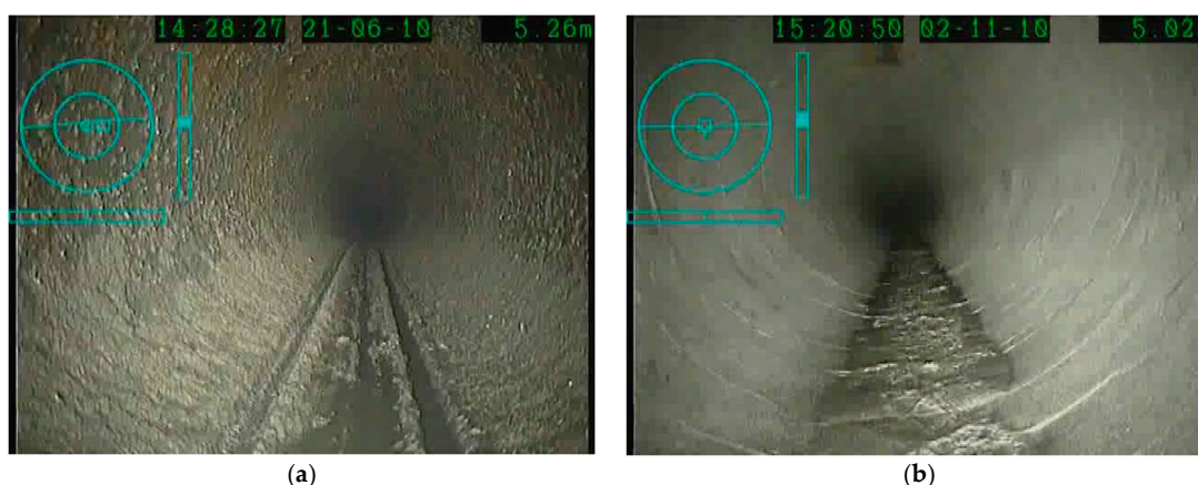
Figure 33. Photos inside the pipe to show the flushing effect in this case study: (a) before flushing; and (b) after flushing.
