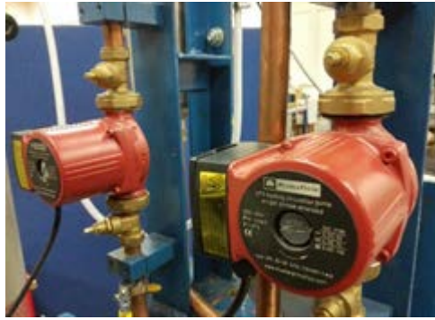
Figure 6.14 The pump employed in circulating system
