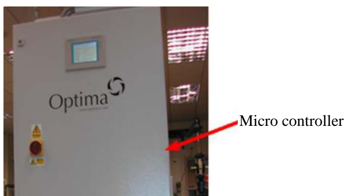
Figure 6.3 Siemens Micro Master Controller system
