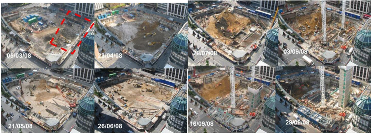
Fig. 6. Snapshots showing the construction sequence (DD/MM/YY). Marked in red is the FE (finite element) analysis area of study (date: DD/MM/YY).
