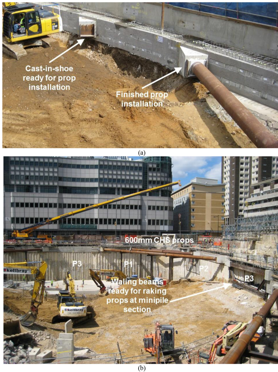
Fig. 5. (a) Prop-wall connection details, and (b) Propping system on 21 July 2008 in the north-east corner.
