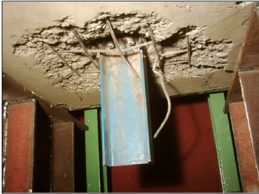
Figure 28 Perforation of the I-section in Slab S1 (Izatt et al., 2009)
