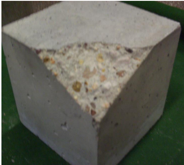
Figure 9: Damages of concrete prepared from cement CEM I 42,5 R after a thermal load of 400 °C
