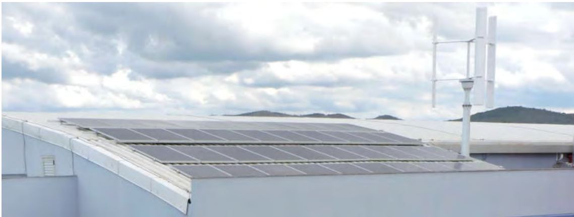
Figure III.2: Photovoltaic panels and vertical axis turbine in the HRGS installed at Unifei (Itabira, Brazil).
