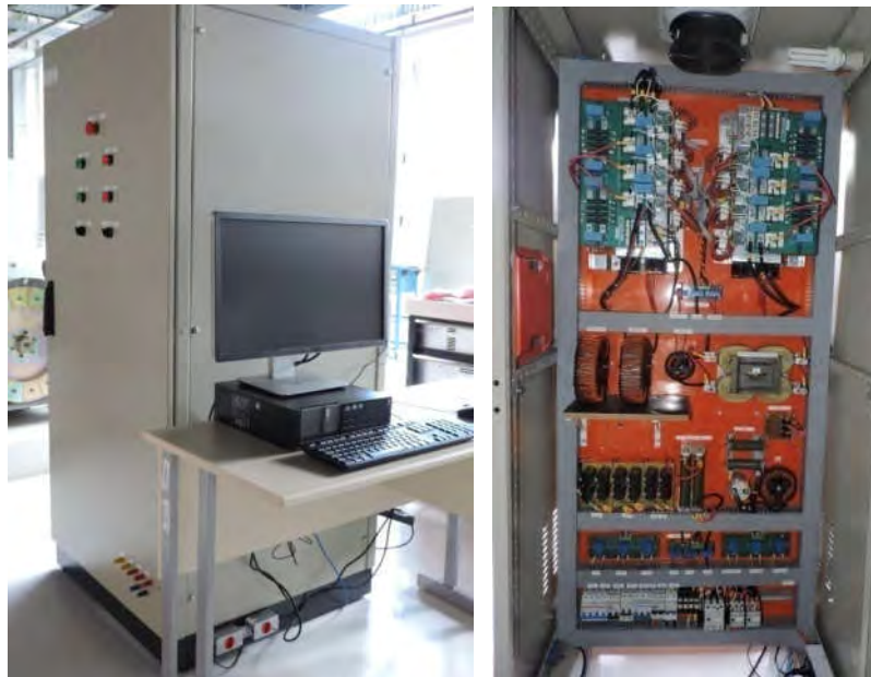
Figure III.3: Converter cabinet of the HRGS.
