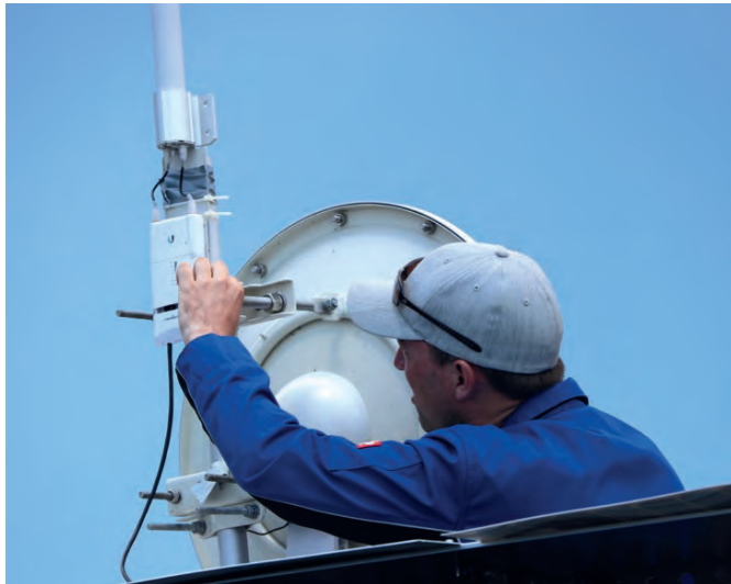
Only if the antennas are exactly aligned can the communications between the lander, the rover, the sensor unit and the control centre function correctly.
