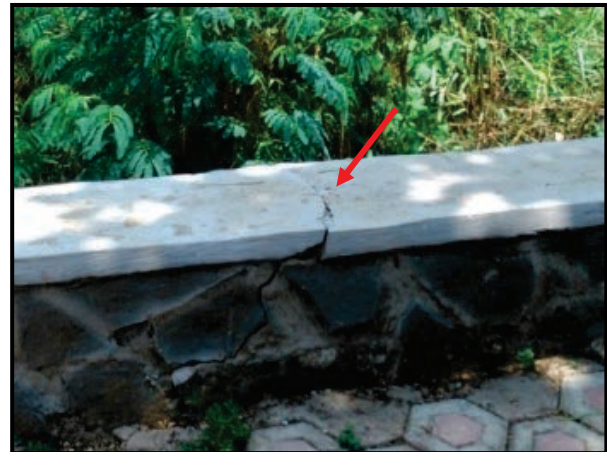
Figure 19. Cracks on the bridge as a manifestation of ground movement due to fault structures in the study area
