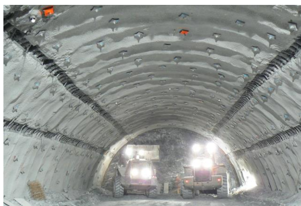
Figure 9. Use of yielding elements in the Tauerntunnel, Austria (Photo: Vergeiner)
