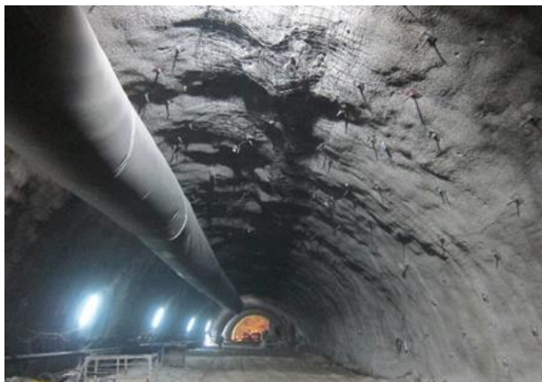
Figure 1. Typical shearing of shotcrete lining along slickenside (Rohtang tunnel, India)
