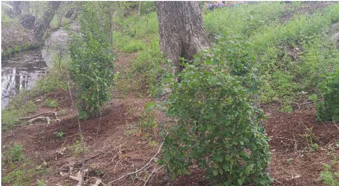
Fig. 3. Hilton Creek streambank at the Botanical Gardens of the Ozarks, Fayetteville, Arkansas shown 5 April 2016 post-restoration, after the 3 April 2016 planting day.
