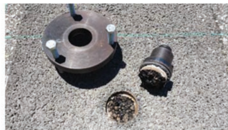
(b) Substrate failure (test strip, field)
