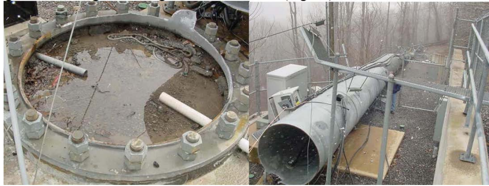
Figure 2.8 Antenna Tower Collapse [12]
