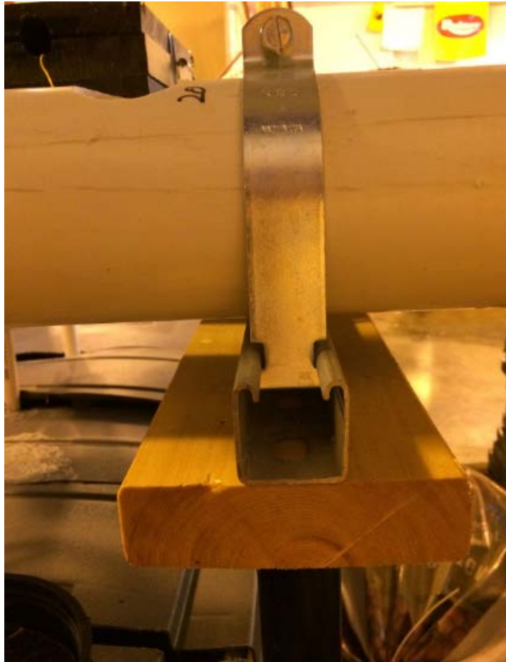
Figure 3.7. Attachment of PVC pipes to support system using PVC clamps, strut channel, and wood board.
