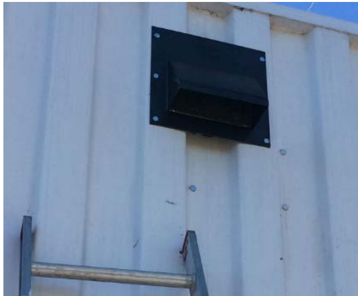
Figure 3.17. Exhaust mount on exterior of shipping container.
