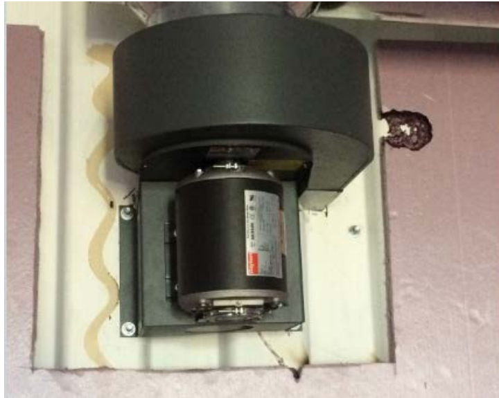
Figure 3.16. Ventilation fan mounted to rear wall.
