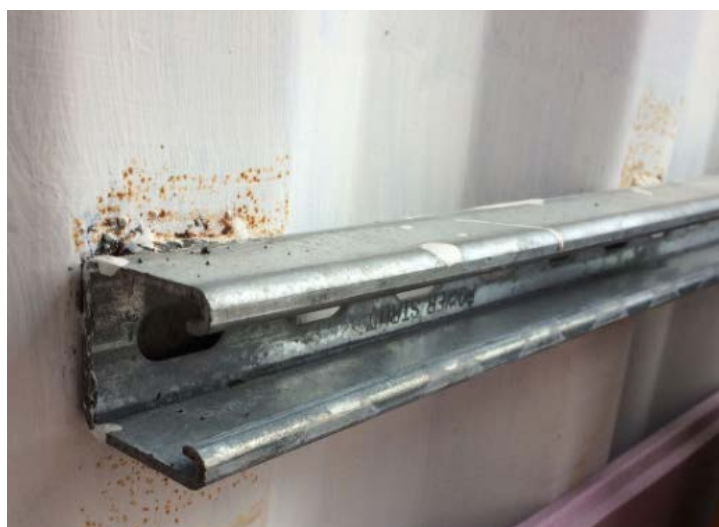
Figure 3.2. Close up of the 1.5" B-line strut channel used for universal attachment points.
