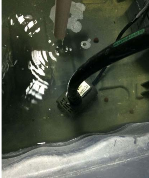
Figure 3.10. Pump and black tubing of irrigation system.
