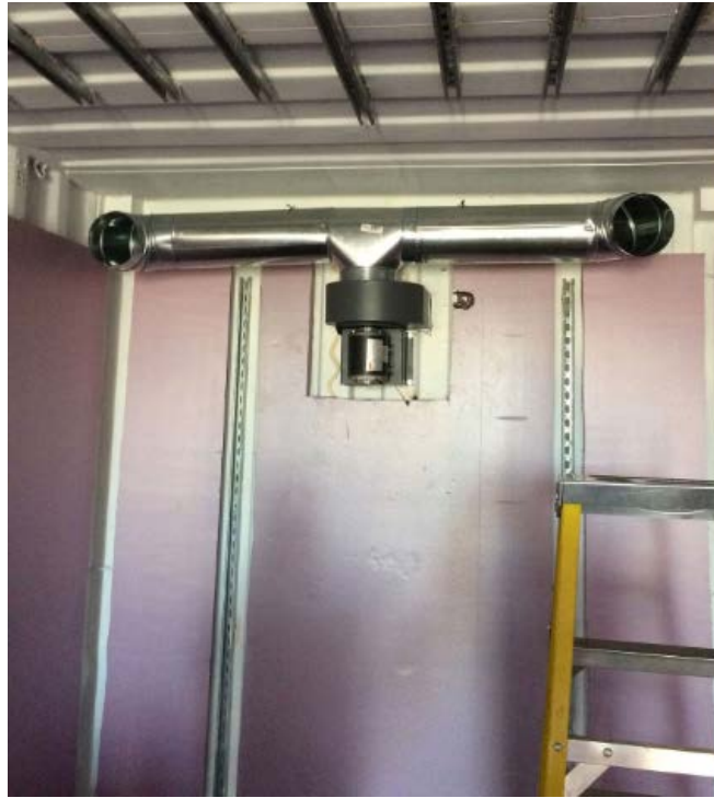
Figure 3.18. Ventilation ductwork and fan on rear wall.
