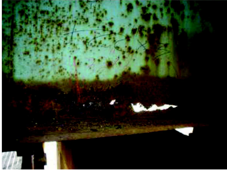
Figure 4.1: Damaged steel girder due to extended corrosion (Zaffetti, 2010)
