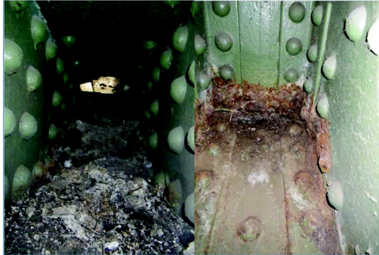
Figure 4.3: Interior of lower chord from truss. Before (left) and after (right) cleaning and washing (Berman et al., 2013)
