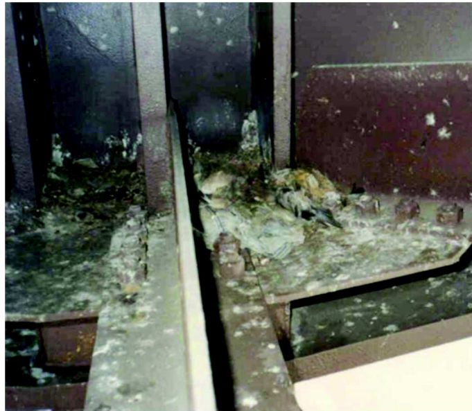
Figure 3.6: Debris accumulation at a steel superstructure connection point (Kogler, 2012)
