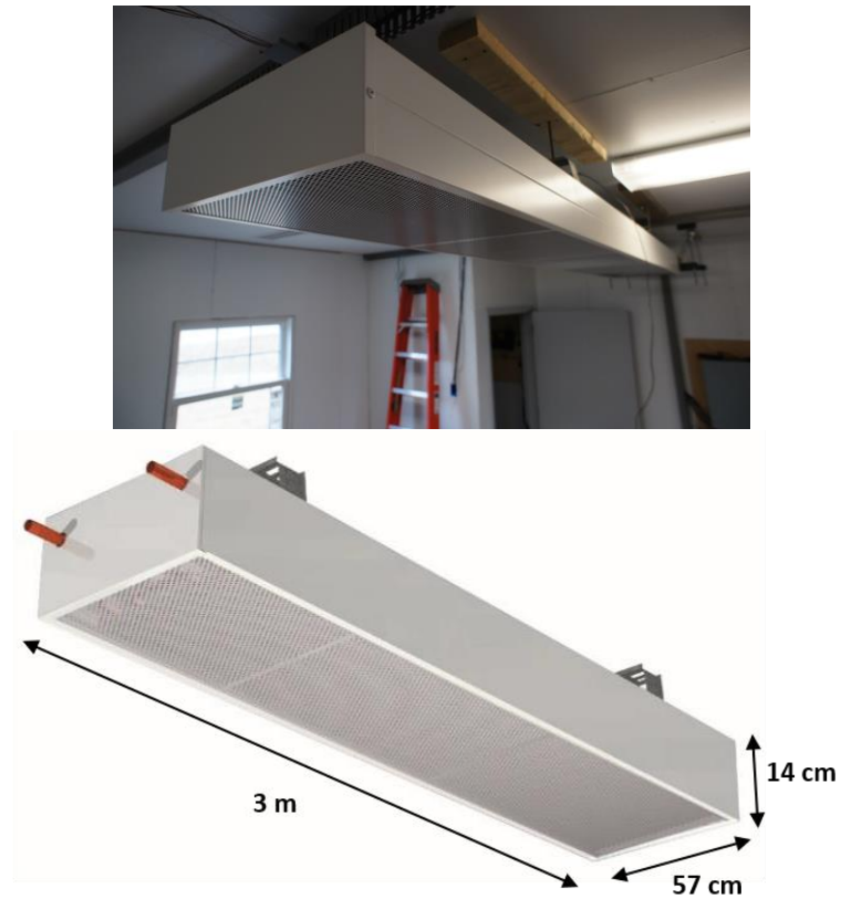
Figure 3-6. Installed passive chilled beam and its dimensions in Bowen test bed.
