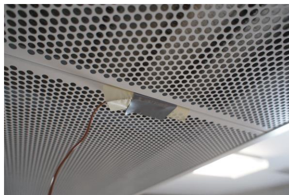
Figure 3-7. Thermocouple attachment on the surface of passive chilled beam.
