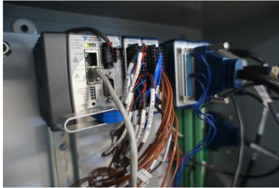
Figure 3-10. Data acquisition device.
