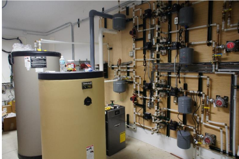
Figure 3-5. Mechanical room at Bowen Laboratory.
