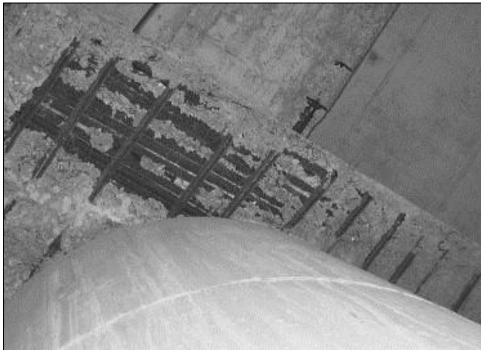
Figure 1-2: Honeycombing as a result of reinforcement congestion [from Kenai and Bahar (2003)].
