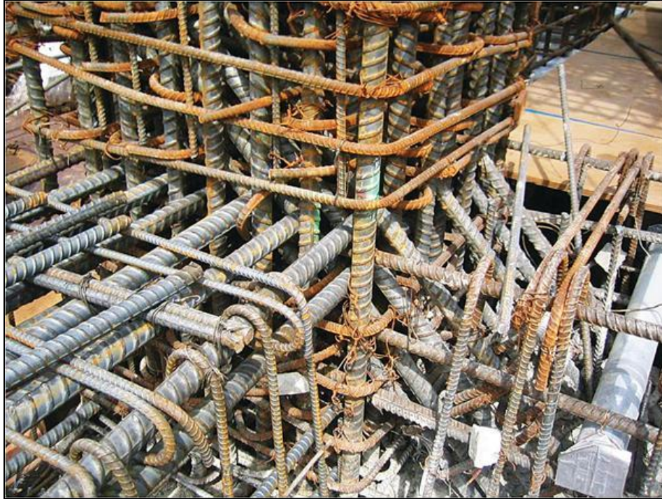
Figure 1-1: Reinforcement congestion at a beam-column joint [Risser and Hoffman (2011)].
