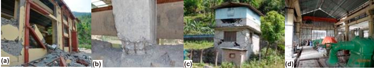
Fig. 35. Earthquake induced damage to the power station (a) wall collapse on riverside (b) rupture of reinforcement bar (c) operator's camp at headworks and (d) machine floor.
