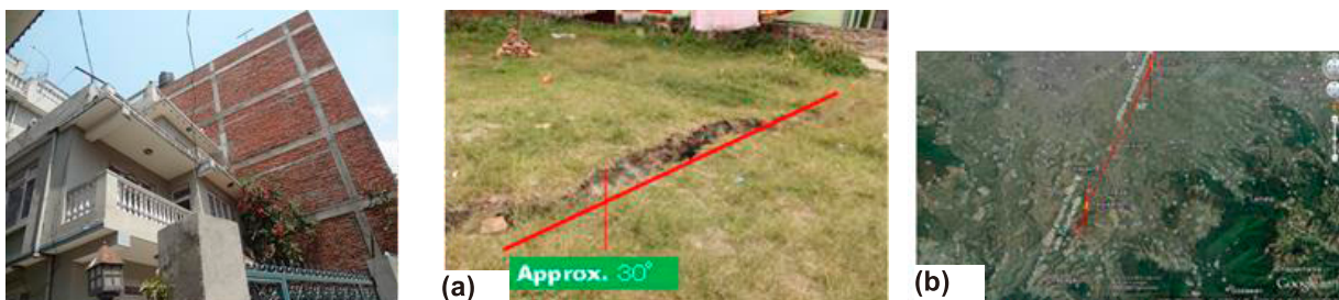
Fig. 10. Settlement and tilting of buildings resulting from ground fissuring.
