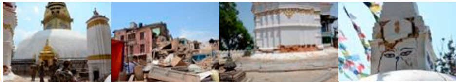
Fig. 24. Damages in Sayambhunath temple complexes.
