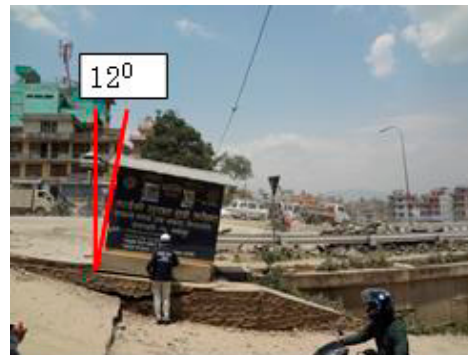
Fig. 6. Slope failure in the Kathmandu side.
