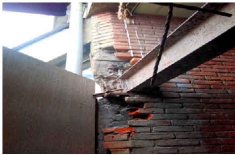
Fig. 8. Concrete spalling and exposure of reinforcement in column..
