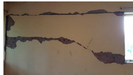
Fig. 7. Cracks seen in masonry infill wall.
