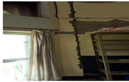
Fig. 9. Cracks in column and adjoining masonry infill wall.
