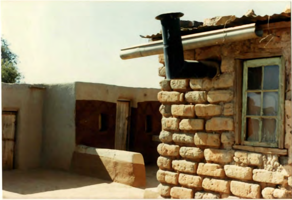
Illus.63. Note the makeshift gutter
