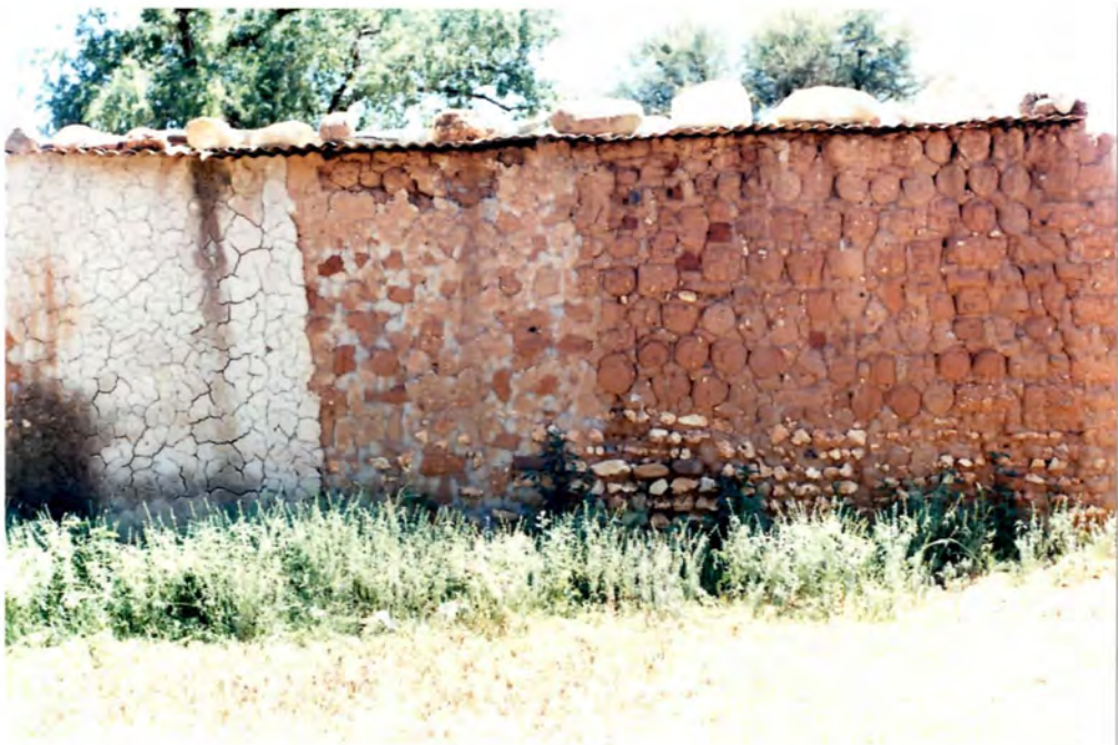
Illus.19. Several rows of stones strengthen the lower part of the wall
