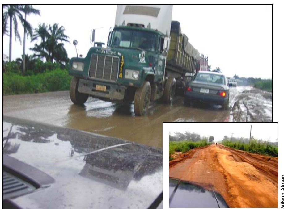
Plate 1: 5-4: Collapsed infrastructure—Port Harcourt-Abak and ( inset ) Ikot Ekpene-Calabar Highways in 2003
