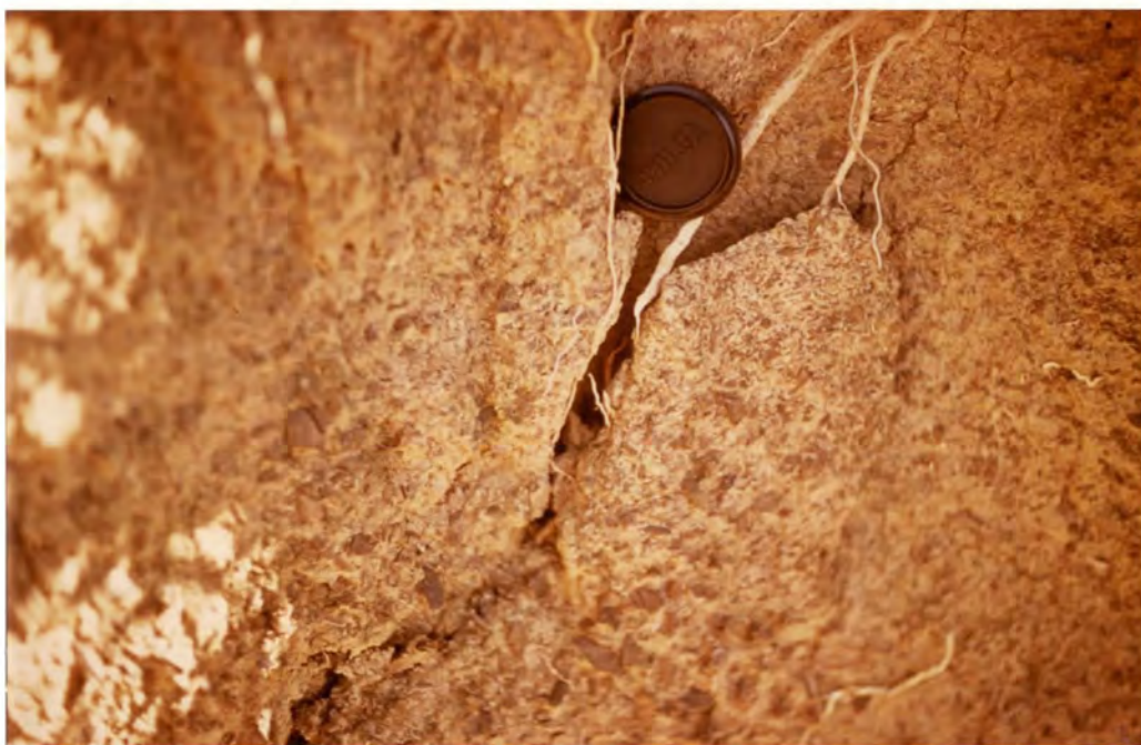
Plate 7.1a. A section of the channel bank at the tributary gully site before an episode of bank collapse.
