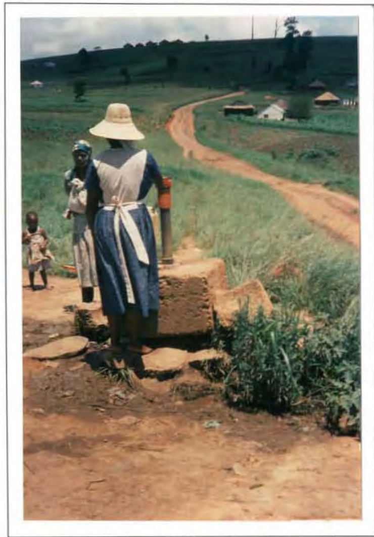
Plate 3. Undermining of the concrete block increases the risk of surface water contaminating the groundwater from which the borehole is drawing.
