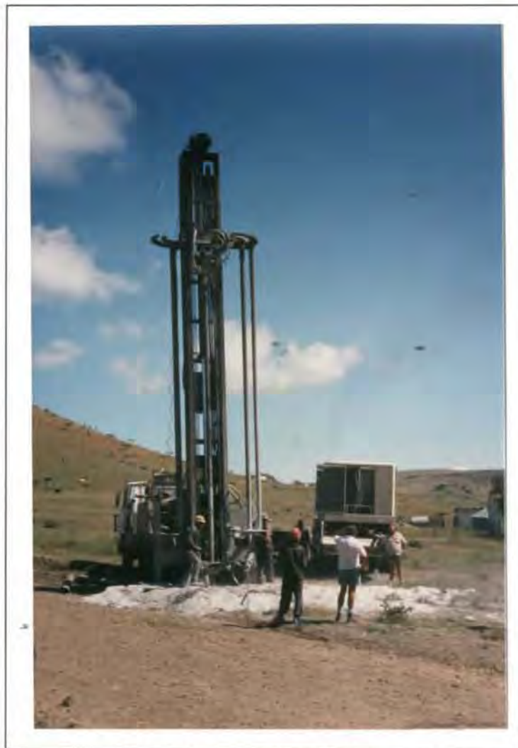
Plate 8. An air percussion rig in operation. Note the air compressor to the right of the drilling rig.
