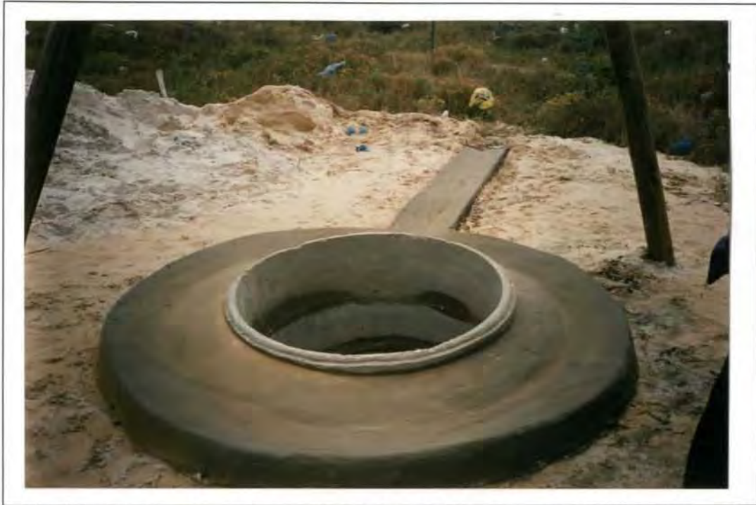
Plate 10. A prototype hand-dug well on the Zululand coastal plain with a suitably constructed concrete apron and channel. Well head protection is still to be placed upon the top rings as shown in Figure 35.
