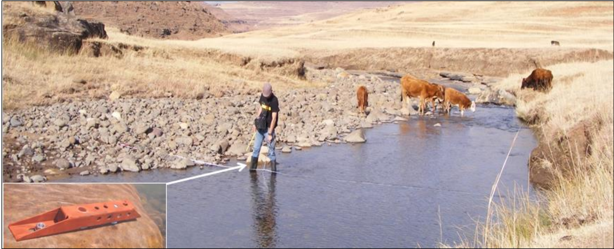
Figure 7.3: Hydraulic site VT1 and underwater image (bottom left) of the level sensor within a metal casing bolted to a large boulder.
