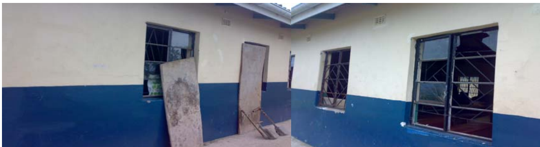
Picture 6.5 Broken windows in rural schools
