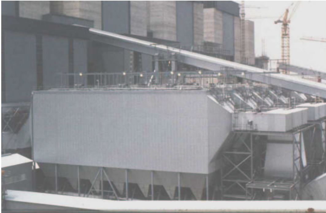
Plate 3.2 : Side view of Lethabo ESP Unit Casings
