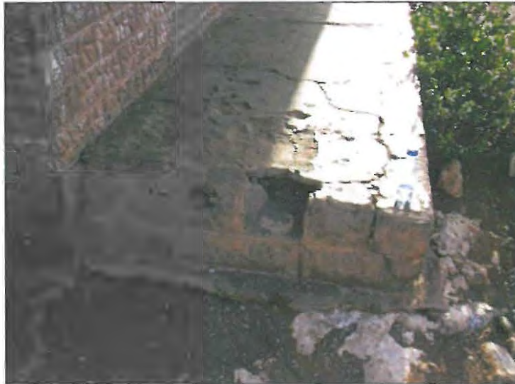
Photo 5.3: Floor slab and block at the Gasehubane Primary School. Note the deteriorating concrete slab and block. The soil in the foreground is contaminated with crocidolite fibres. (Photo by author)
