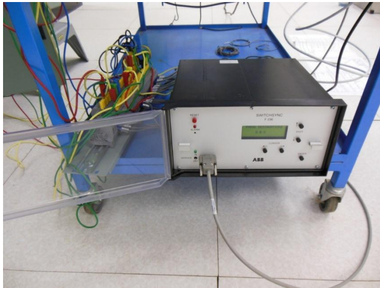
Figure 8: ABB F236 wired into the closing circuit of Transformer 1 at Dedisa substation
