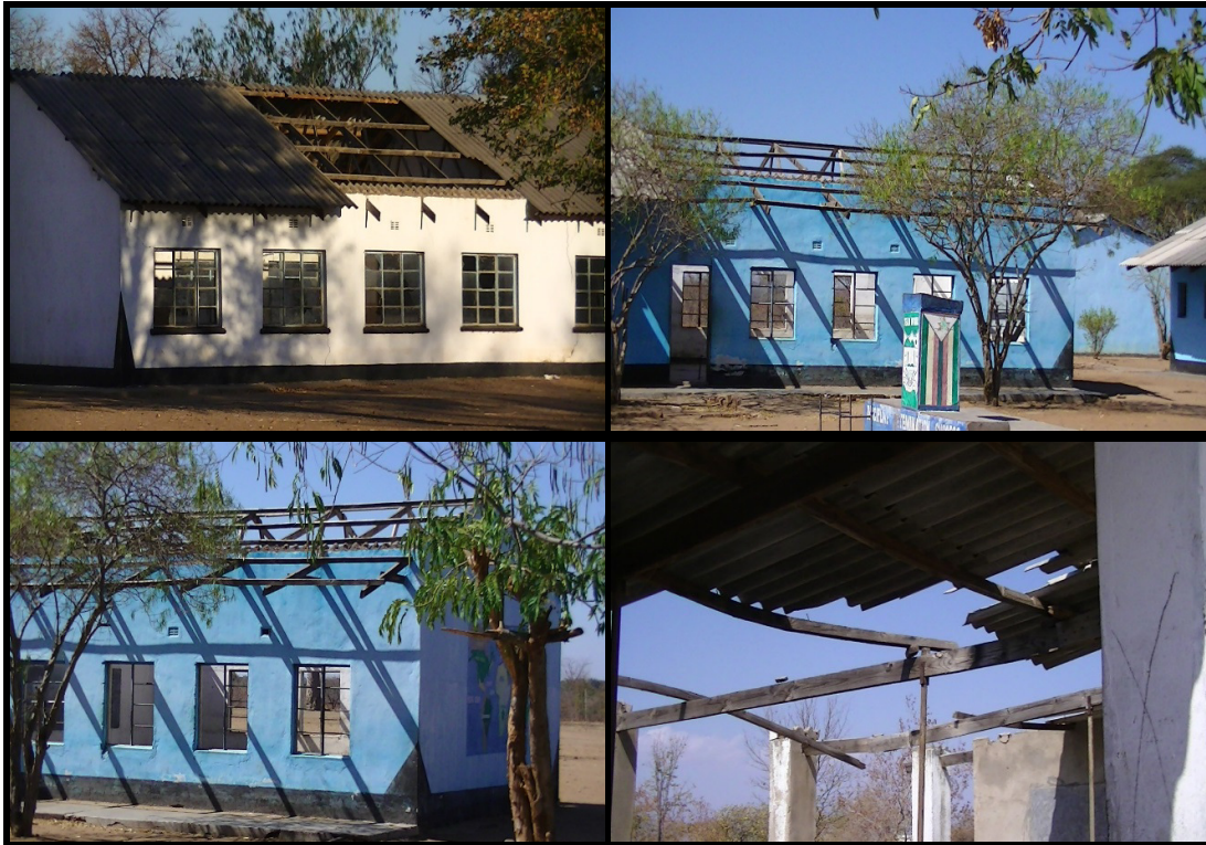
Plate 5.1 Structural damages caused by violent winds in Muzarabani
