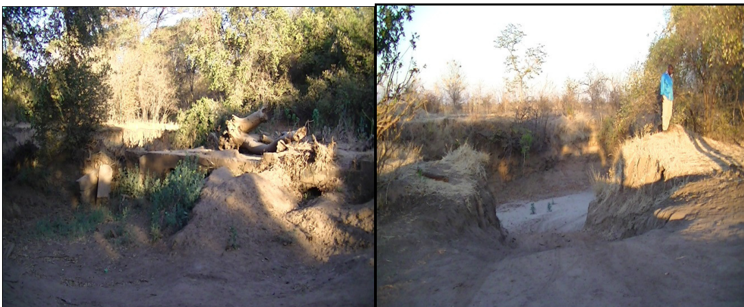
Plate 5.2 Structural damages by floods in Muzarabani
