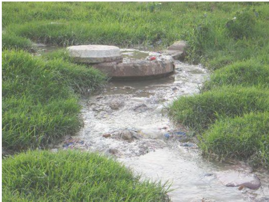
Figure 6.2: A sewerage leak flowing into the upper catchment of the Bloukrans River near Nathaniel Nyaluza School during 2013.
