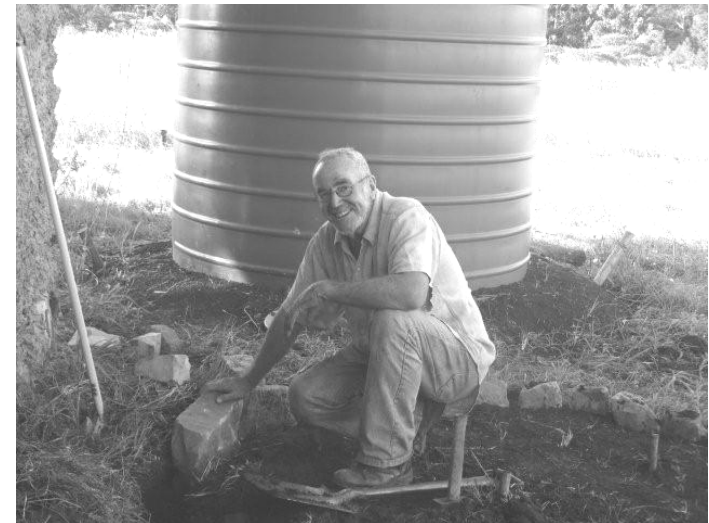
Tim Wigley placing a circle of stones round a tank to begin making a base
