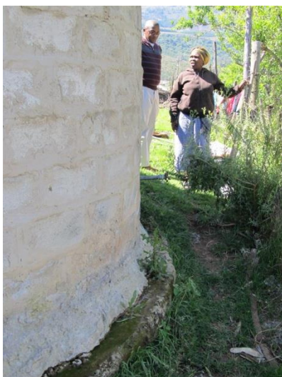
Figure 5.28: Sisiwe shows her leaking cement reservoir (Cata, 2013)
