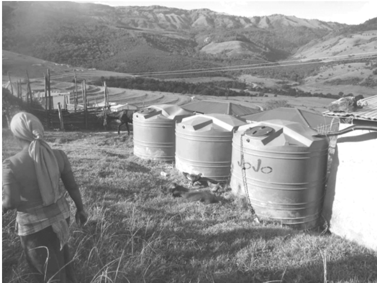
Tanks storing rain water collected when it flows over the ground. Note: to get the top of the tanks lower than the catch pit it was necessary to partially bury the tanks
