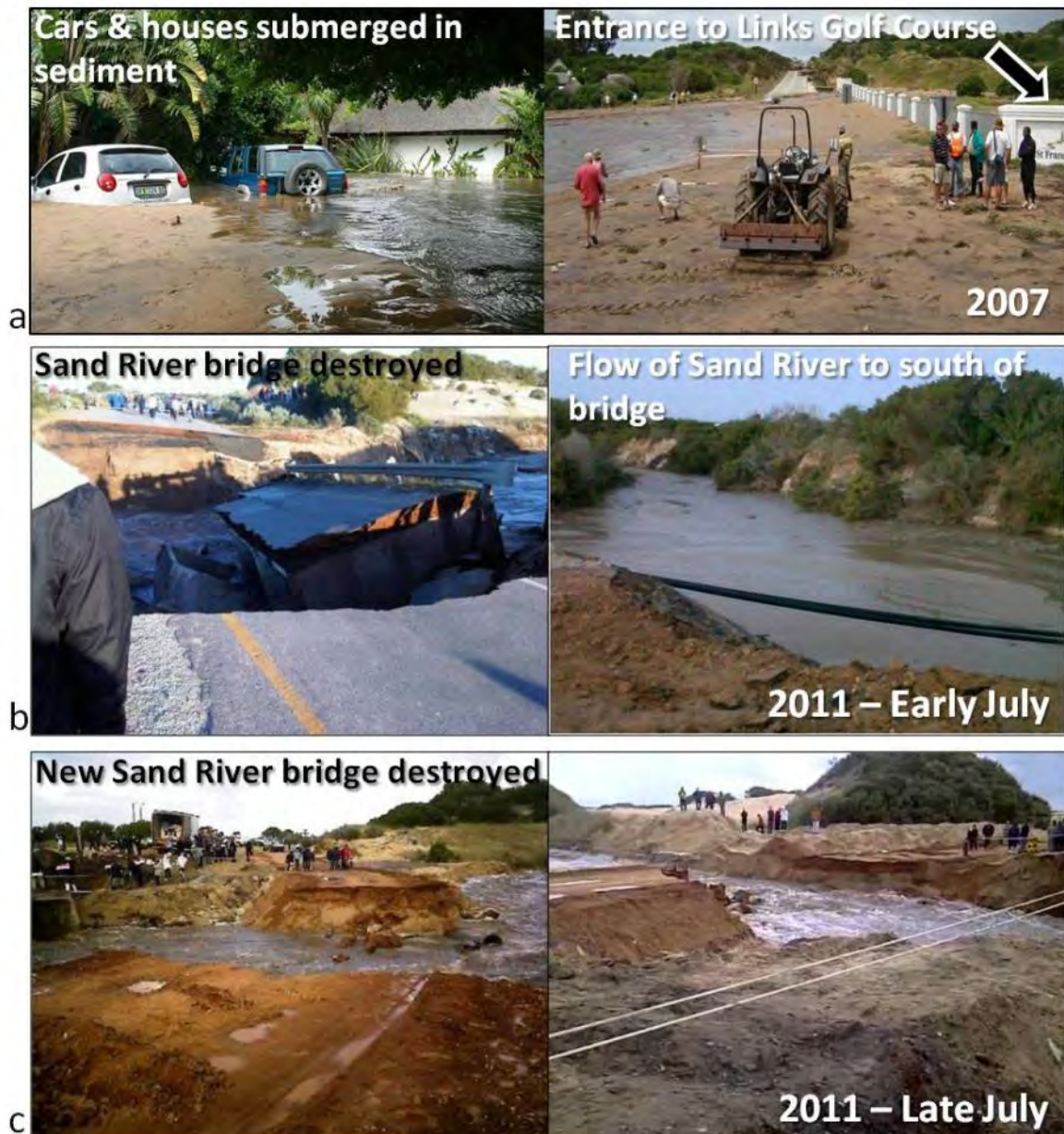
Figure 6-11 (a, b & c): The destruction caused as a result of floods and/or debris flows largely related to extreme and intense rainfall events. a: massive flood event over Links Golf Course 2007, b & c: debris flows destroying the Sand River Bridge across the R303 in 2011.
