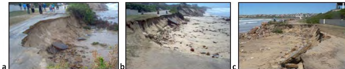
Figure 1-3 (a, b & c): Erosion of Ralph Road along the St. Francis Bay shoreline. Photographs 2a and 2b were taken 24 hours apart in March 2007, during which time the width of the road was reduced by erosion.
