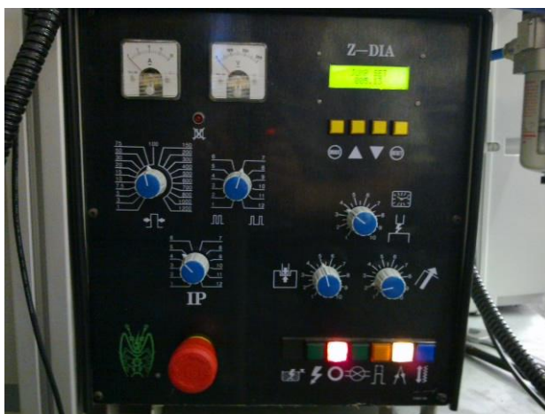
Figure 3.2 Front Panel of Alic-1 Power-Pack/Controller
