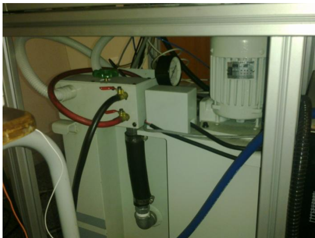
Figure 3.3 Dielectric Fluid Tank and Pump of Alic-1
