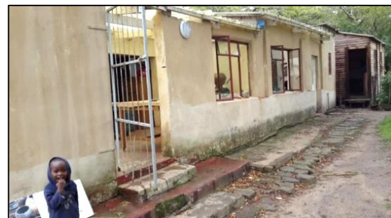
Fig 4.7: The Front View of Studio 2 gate indicates the rusted and broken burglar gate used to secure the building. The wooden printmaking studio is visible in the background of the photograph, source H. Osner.
