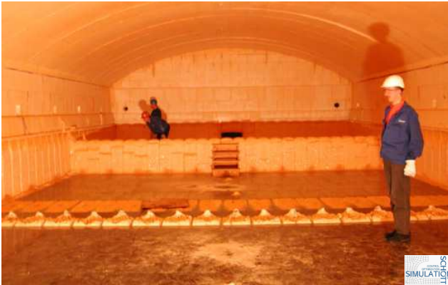
Figure 7.1: Glass melting tank after cooling down.
