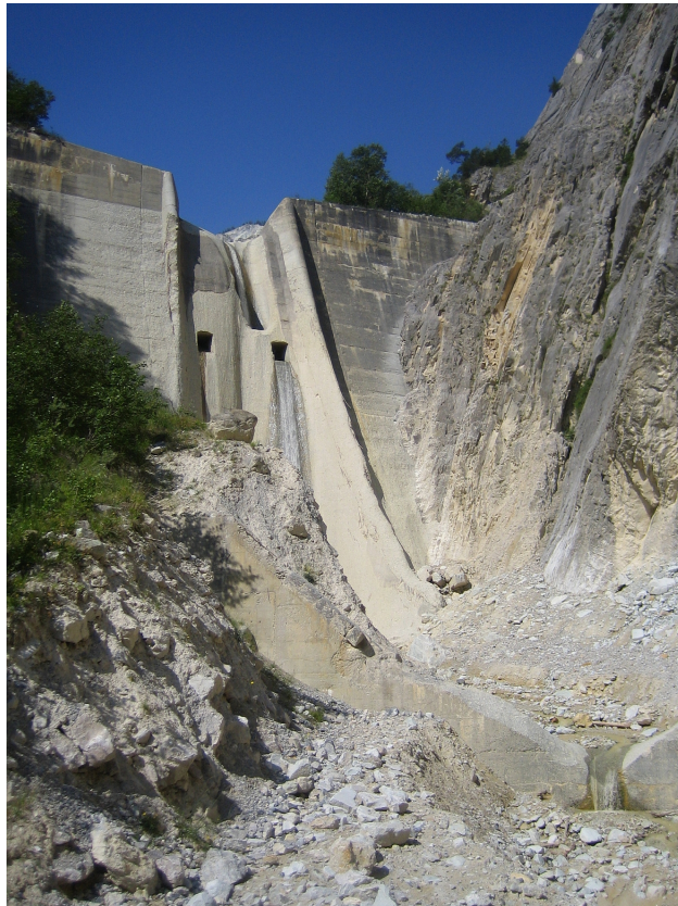
Figure A.4: The sediment retention dam (CD1) seen from downstream, total height is 40 m. Note abrasion of concrete structure by debris flows.
