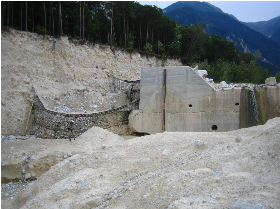
Figure A.12: Deeply incised active channel on the Illgraben fan. Stabilization and protection of damaged check dam due to lateral erosion and bank collapse with ring net barriers.
