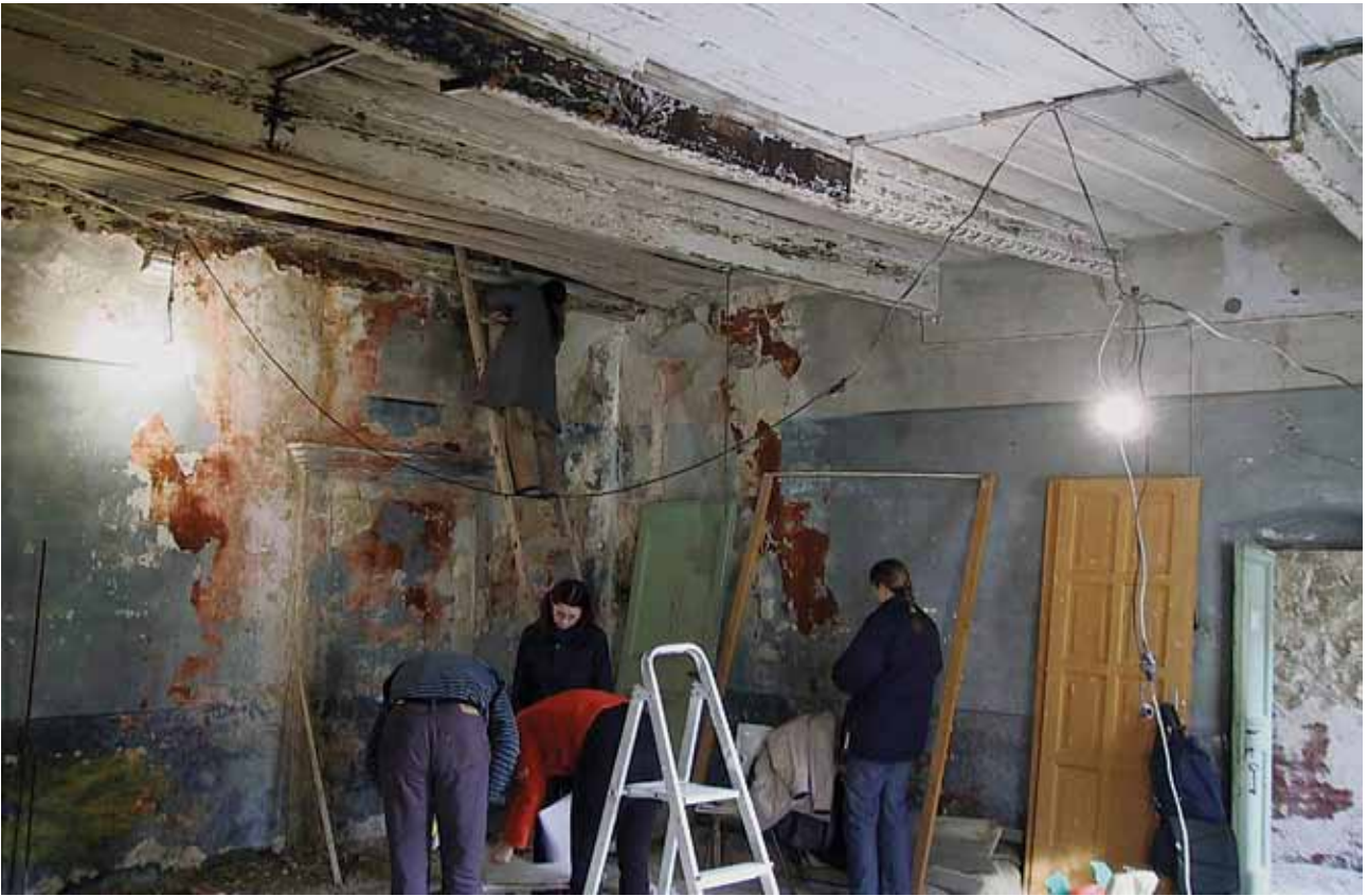
24 Interijer kuće prije radova sanacije i rekonstrukcije (foto: Giuseppe Sava, 2003.) Interior of the house prior to rehabilitation and reconstruction works (photo by Giuseppe Sava, 2003)
