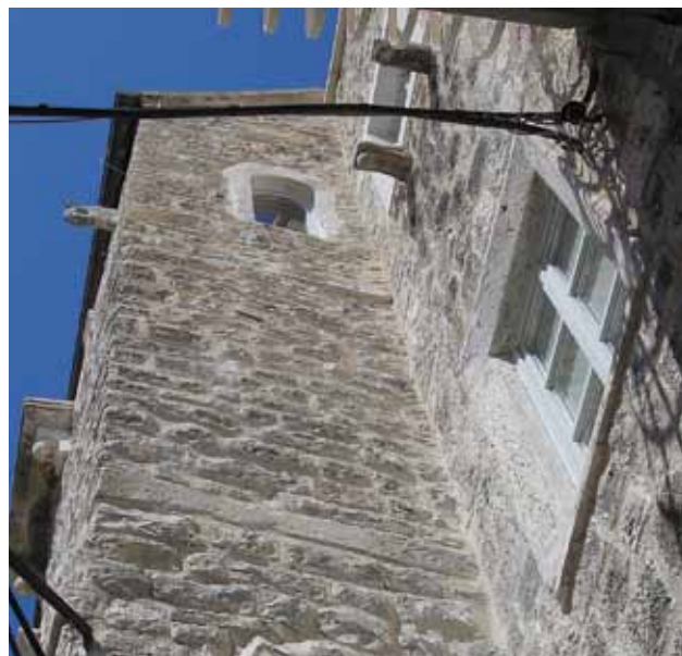
12 Ranogotički prozor na južnome pročelju i ostaci horizontalnih vijenaca, tzv. Markapiana (foto: Anita Gamulin, 2008.) Early gothic window on the south facade and remains of horizontal wreaths, so called, Markapiana (photo by Anita Gamulin, 2008)
