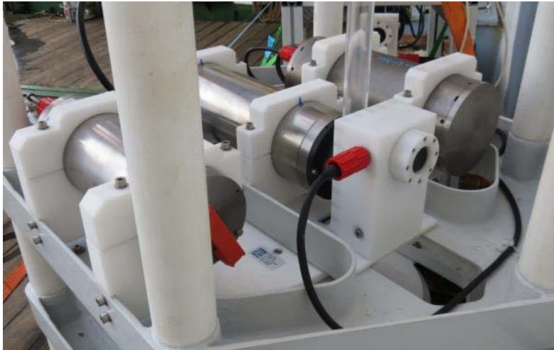
Figure 2: Camera System on BOP with the camera housing (for camera, lens and system electronics), the VIS light source and the Li-Ion battery
