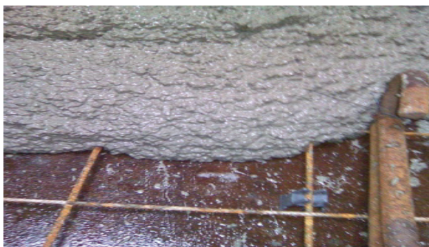
Figure 19 A detail of consistency and deposition of concrete with waste polyurethane foam with reinforcement in the mould
