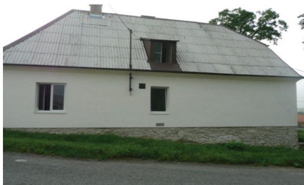
Figure 15 A view of final façade from the west, insulated by means of thermal insulating polyurethane mortar for rendering
