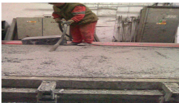
Figure 20 Compaction of concrete with waste polyurethane foam in the mould by an immersion vibrator
