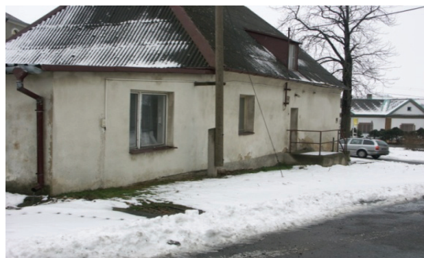
Figure 14 A view of reference building from the west before insulation by means of thermal insulating polyurethane mortar for rendering
