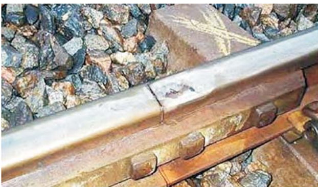
Figure 17 Damaged insulating joint
