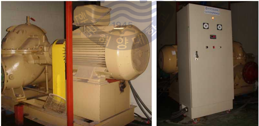
Fig. 3.4 Photo of pump & inverter
