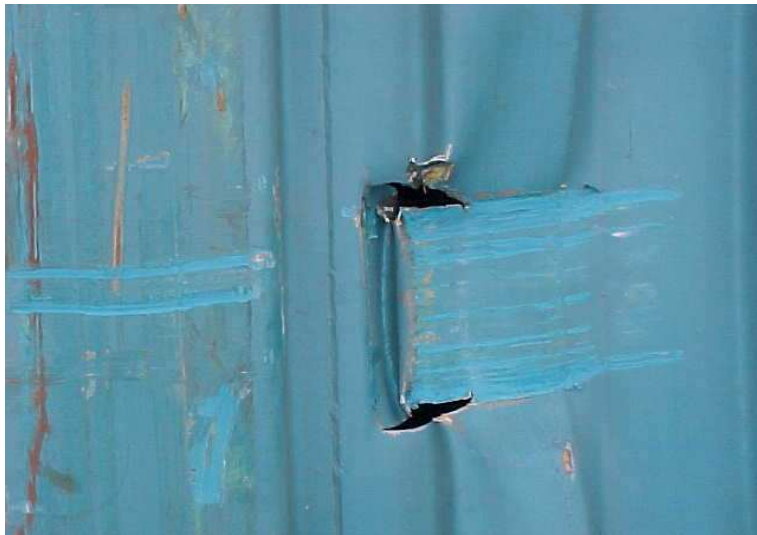
Fig. 3.4 An accident of electrical fault(b)
