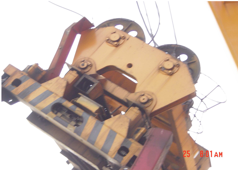
Fig. 3.2 An accident of mechanical fault(b)
