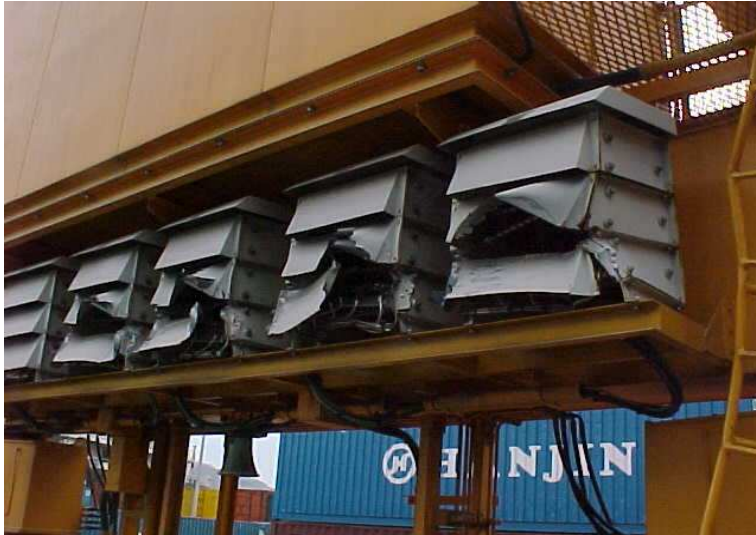
Fig. 3.8 An accident by outside vehicles
