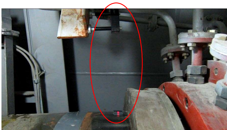
Fig. 8.5 Laser sensor installation
