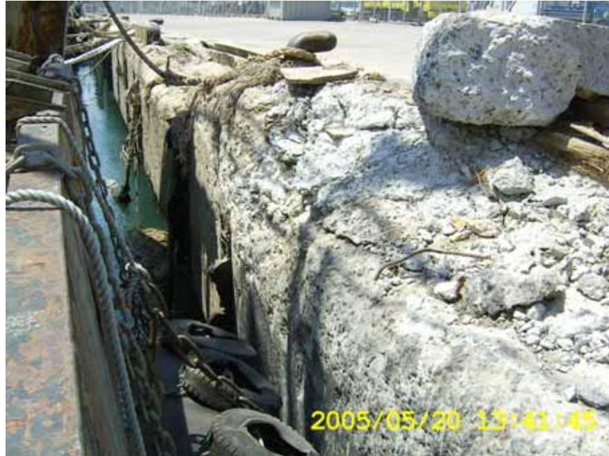
Fig. 2.2 Damaged pier by harbor oscillation
