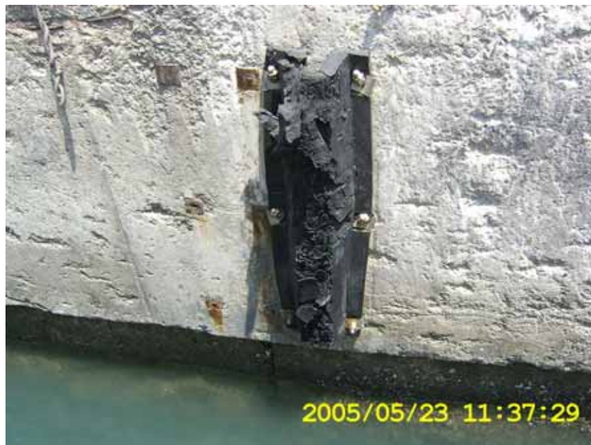
Fig. 2.3 Damaged rubber fender
