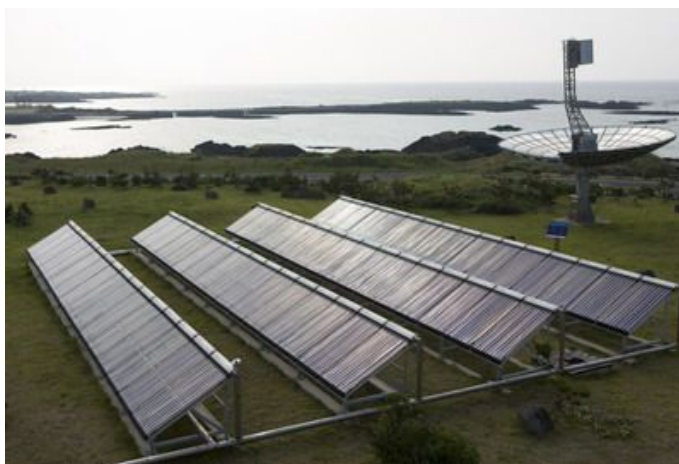
Fig. 2.11 Photograph of solar collectors
