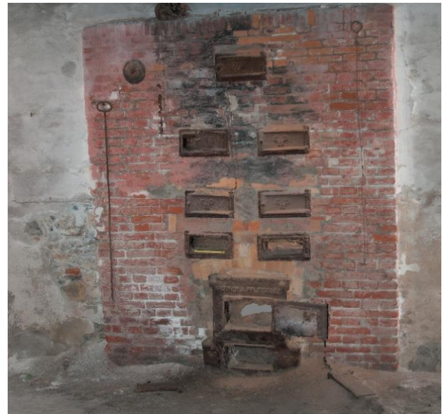
Figure 6. Tiled model view of case C, a wall of the ovens in the kitchen of the Albergo dei Poveri .
