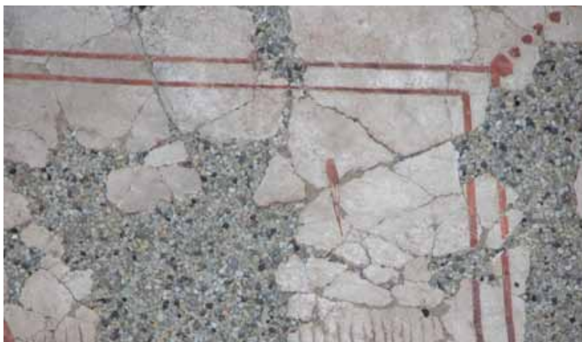
fig. 23 The scratches on the wall-painting (photo by L. Borhy, 2010)
